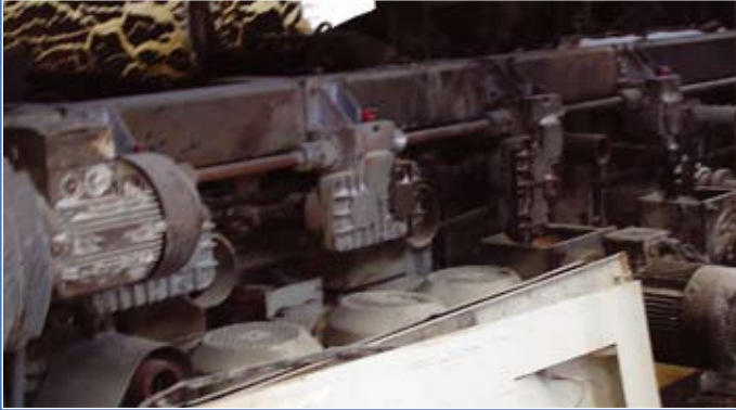
Damage caused by fire
